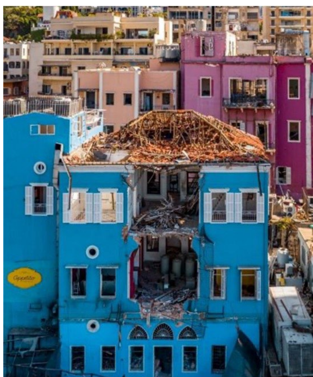
Fig. 2 Three story historical structure of side facing the port.. Photo credit: Rami Rizk.
